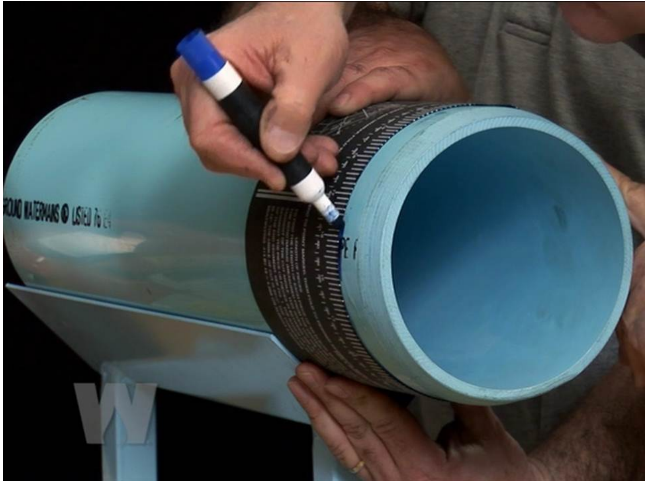
Figure 9 - Mark the pipe about the entire circumference to ensure a square cut
