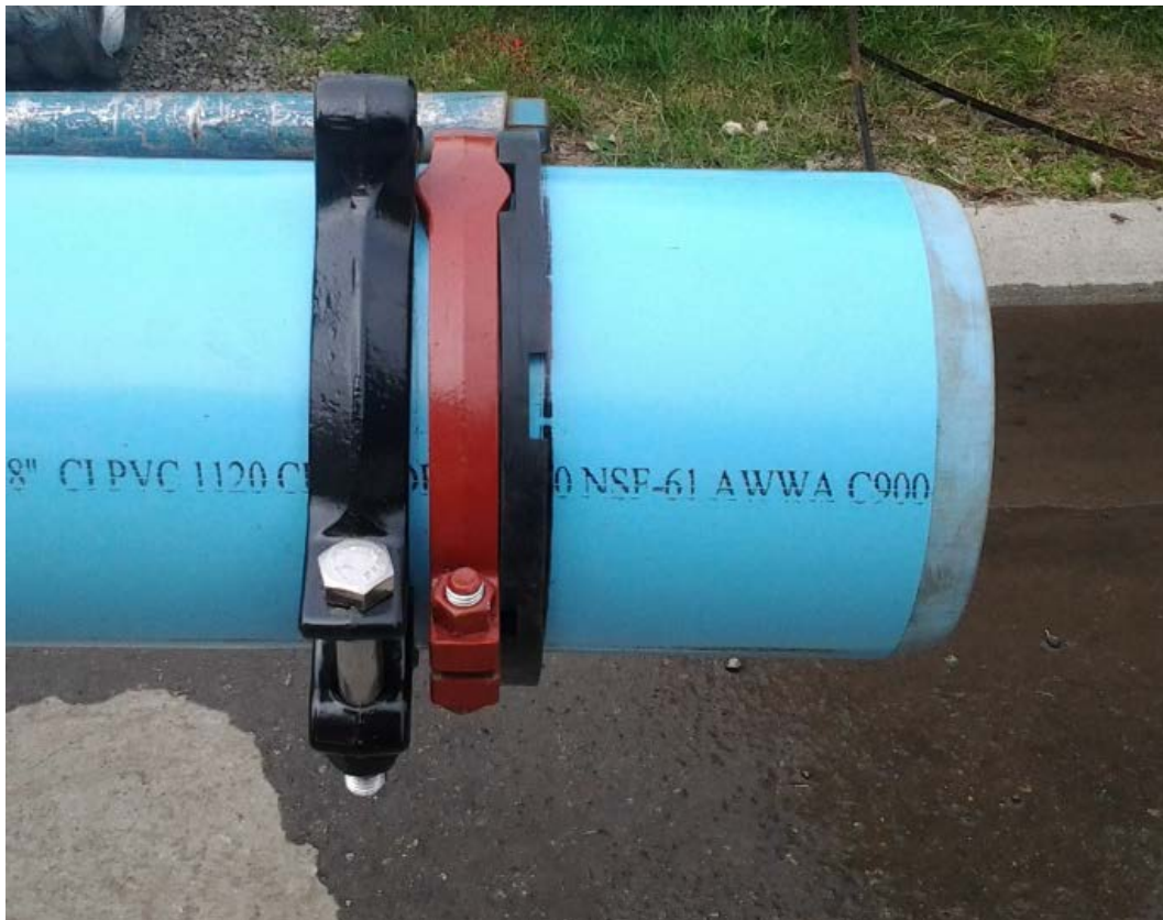
Figure 8 - Series 5000 Mega-Stop™ installed with the insertion line showing. Series 2600 PVC Restraint from EBAA Iron installed in junction for this joint
